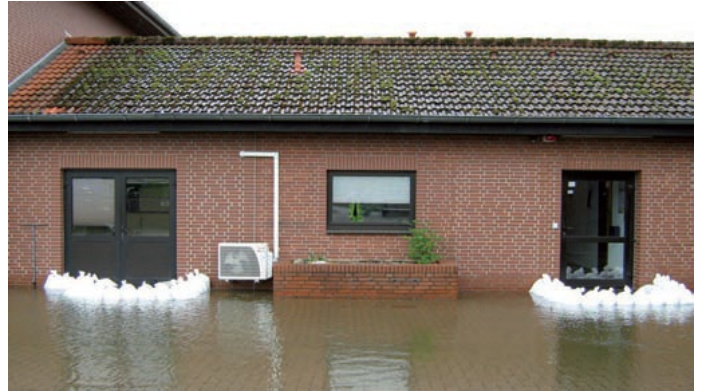
Figure 13: Control room of the treatment plant in Soßmar (Fischer, 2013)
