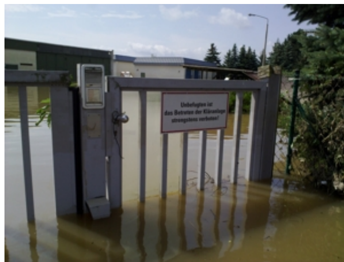
Figure 11: The flooded treatment plant in Zittau (Kuba, 2011)
