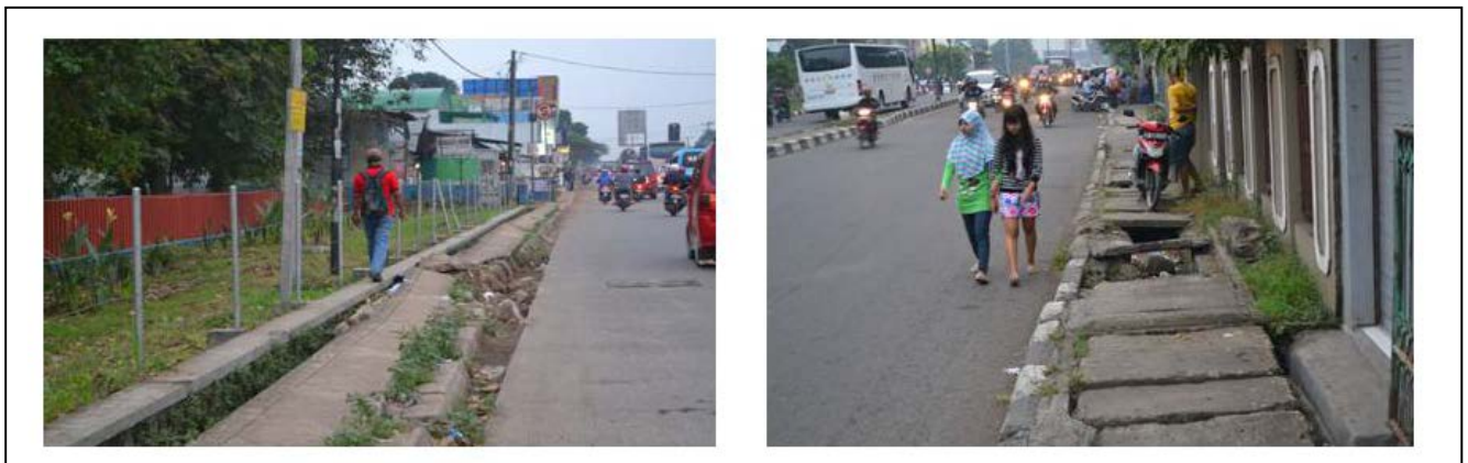
Figure V.7. The Bad Condition of Pavement in Bekasi
