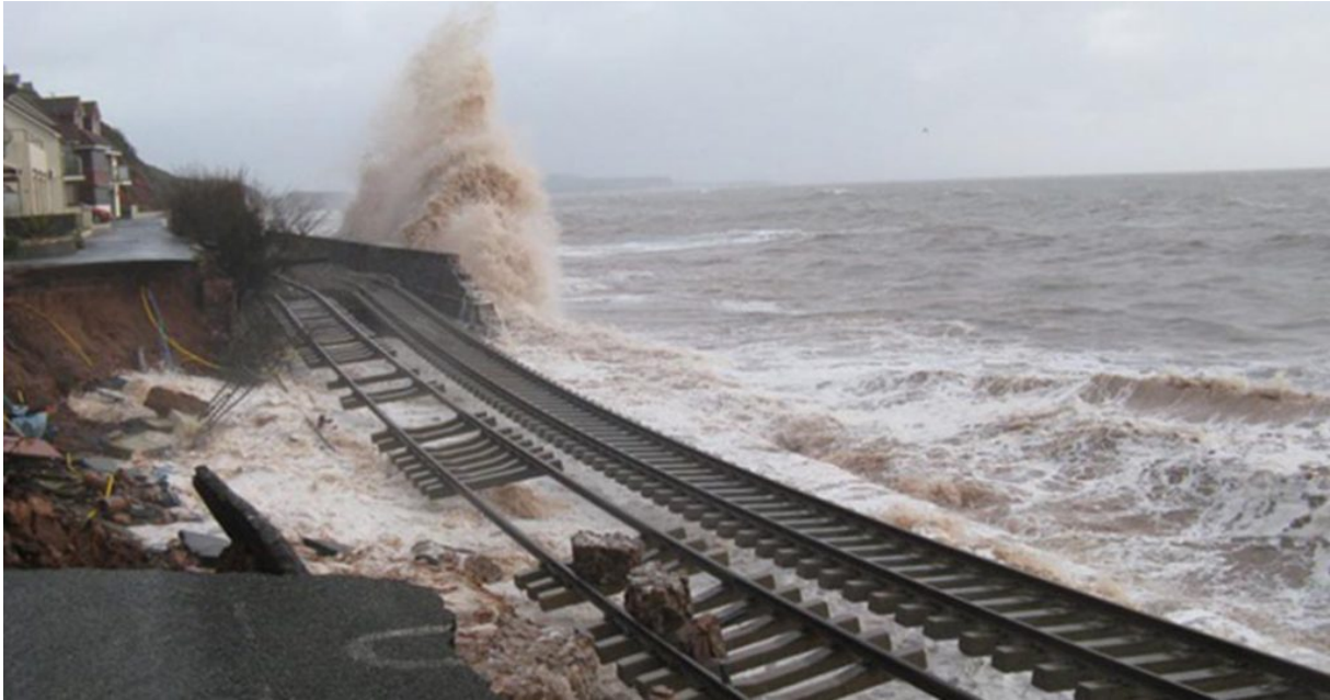
Figure 5: Damage from the 2014 storm in Dawlish closed the line for several weeks. Source: Network Rail
