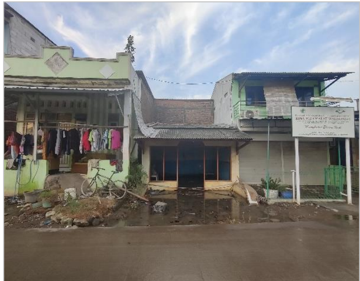
Figure 4.8 A sinking house in Semarang (photo by author)
