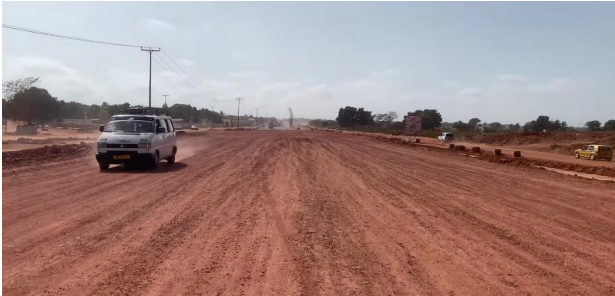
Figure 13: Image showing the current condition of the Bertil Harding Highway, and the diversion route (right side of photo). Source, Nice Gambia, YouTube, 2023.
