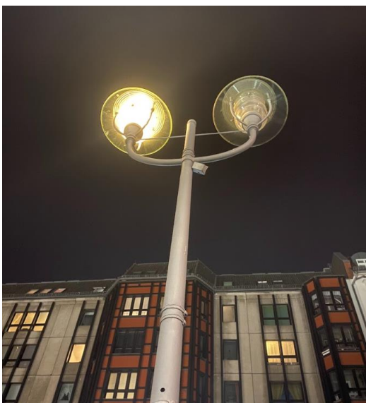
Figure 16 Broken light (Author, 2023)
