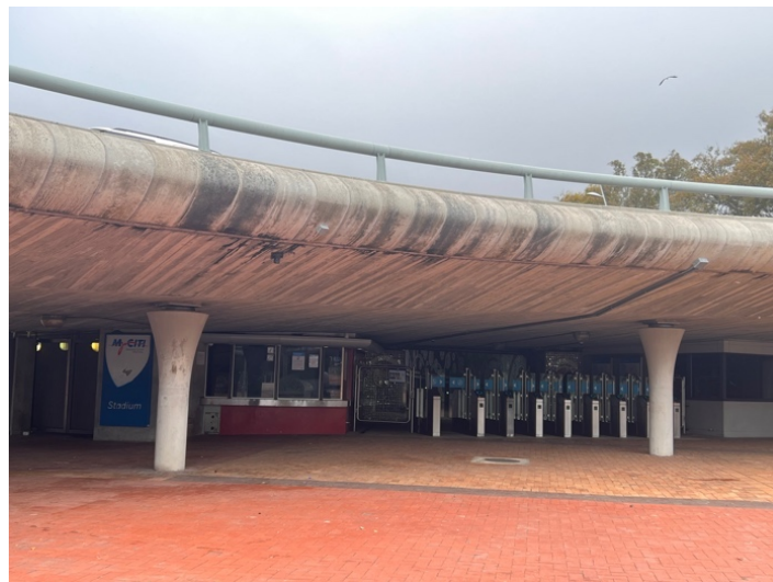
Figure 10: The constructed public infrastructure right next to the DHL stadium (Author photo)
