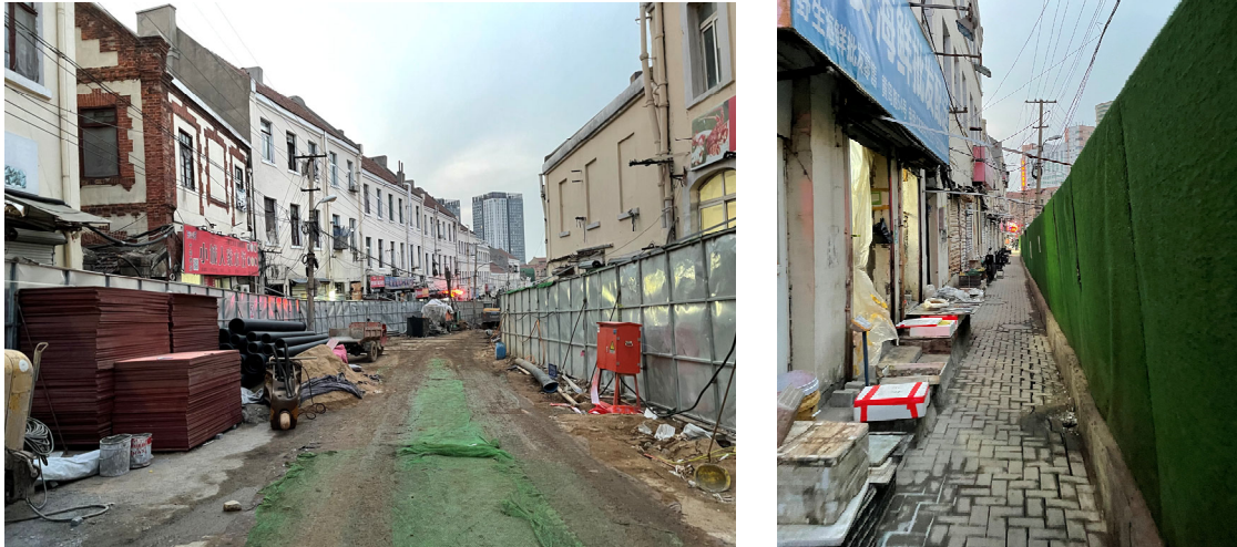
Figure 5: The excavated and blocked part of the street (left) and the remaining unblocked part (right).
