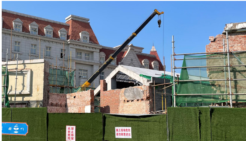
Figure 4: Weixian Road No.19 under renovation. Source: fieldwork photo by the author, February 16, 2022.
