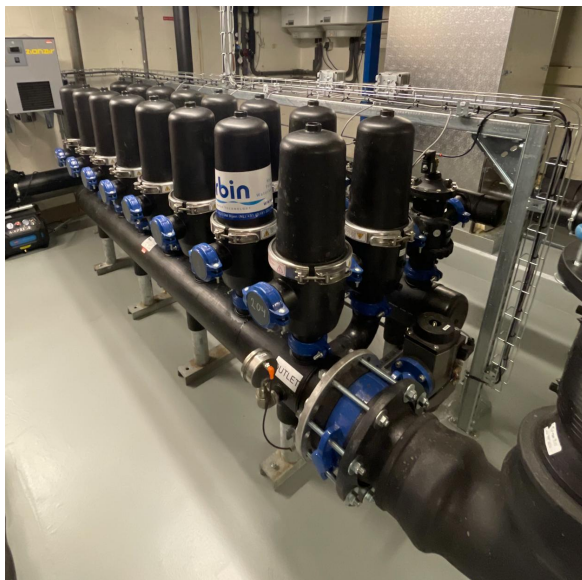
Figure 21: The filtration system
