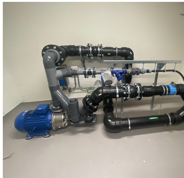
Figure 19: The pumping installation (Author, 2023)
