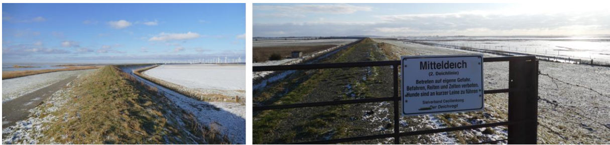
Figure 15: Second dike line or "middle dike" between two polders whereby the older polder lies lower below sea level than the younger one as the older was cut off from sediment input earlier. Source: Author.
