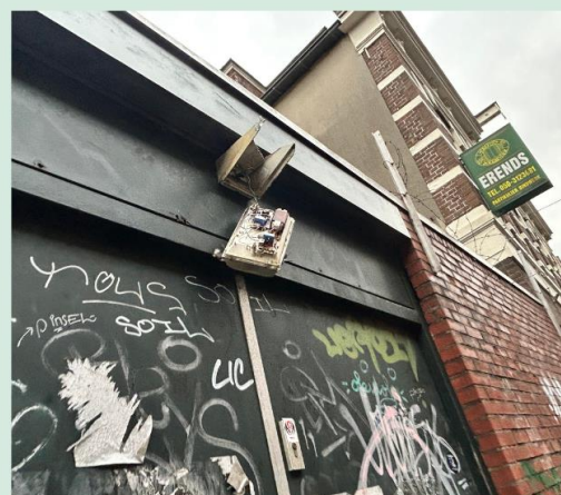
Figure 5: Maintenance issues, vandalism & lack of functional windows
