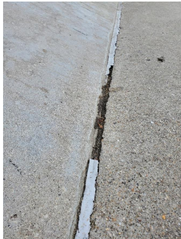
Figure 19: Cracks in the concrete of Skatepark Karding
