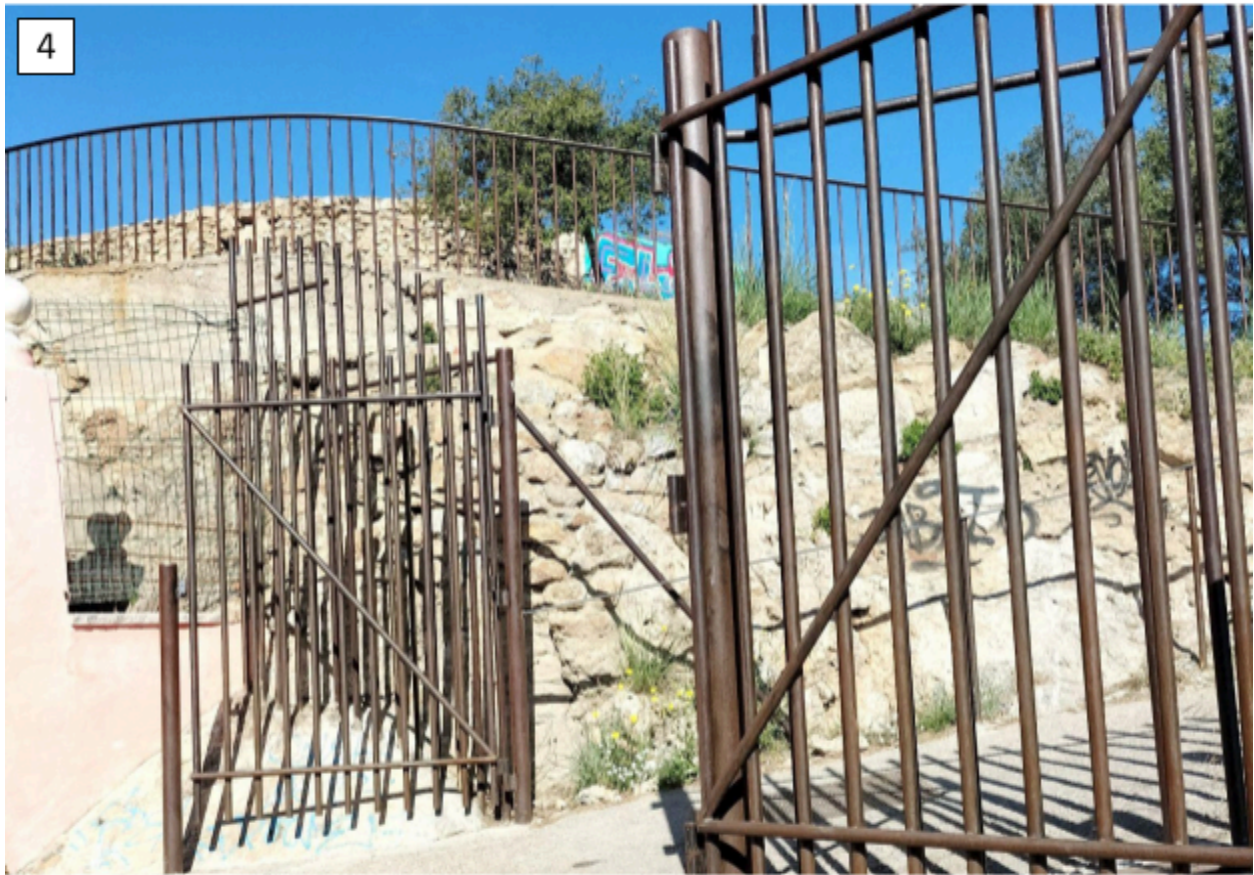
Note: Photograph of one of the entrances to the site. Own work.
