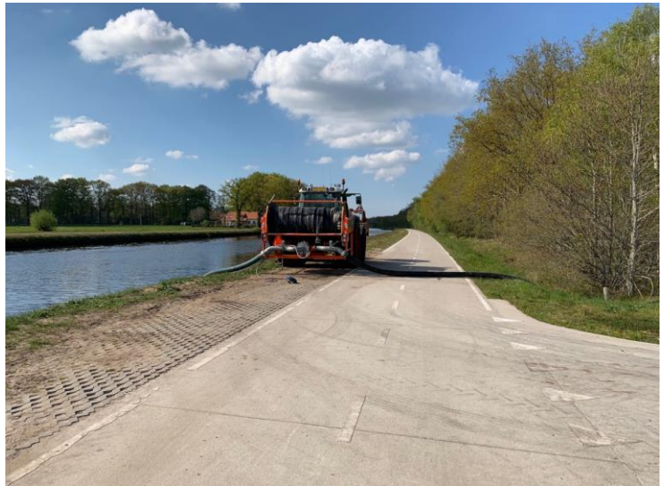
Figure 24: Water pipe blocking cycle path
