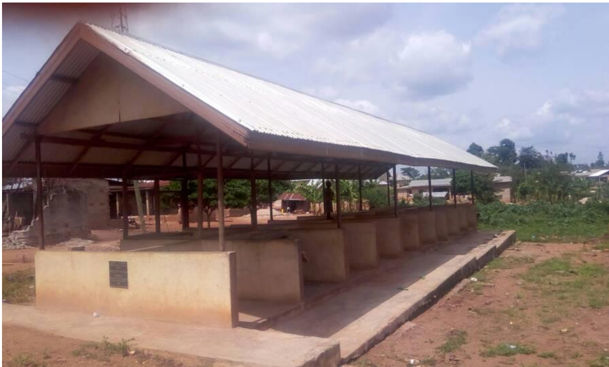
Figure 11: Abandoned market infrastructure in Ejuratia (Source: Field Survey, May, 2017)
